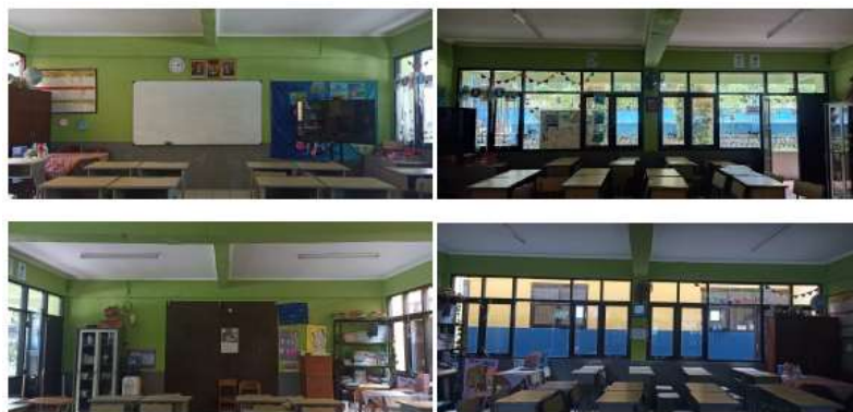
Figure 5. SD A Classroom Condition; Front View (Upper Left); Left View (Upper Right); Rear View (Bottom Left); Right View (Bottom Right)
